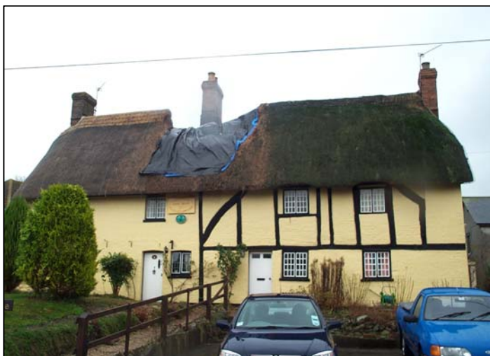
Photograph 9 – damage apparently caused due to an imperfect chimney
