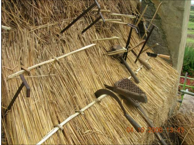
Photo 4 - Close up of combed wheat being laid. The provision of a horizontal bond formed of hazel liggers (which will eventually be concealed – see Diagram 1) highlights a major difference to laying in the Long Straw style. It should be noted however that the bond in most historic buildings within the District is formed by tying a small portion of each bundle to its neighbour – a straw bond.
