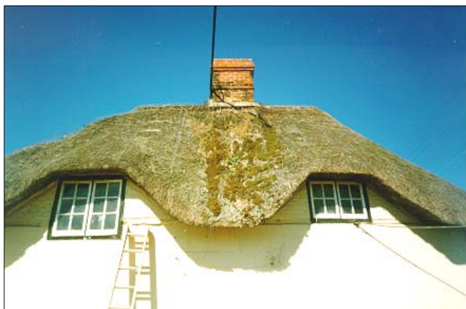
Photograph 1 – Time for action. Note the concave dip and fixing spars visible on the left hand hip, the stranded flashing around the chimney, and the heavy build up of moss indicating permanently damp areas.
